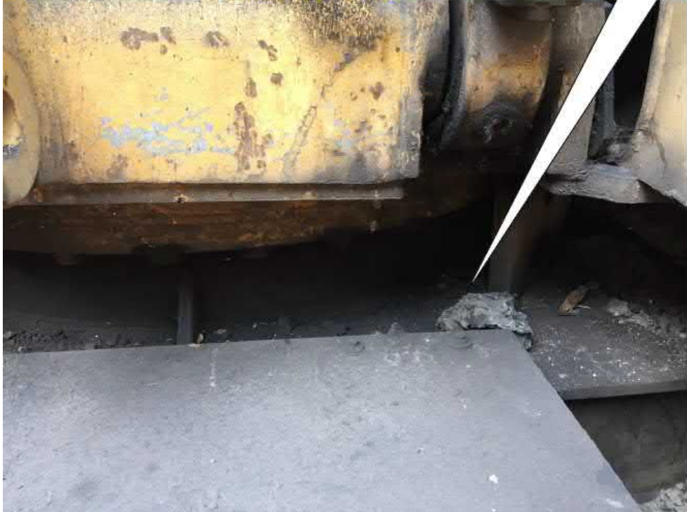
Debris on Exterior Body
