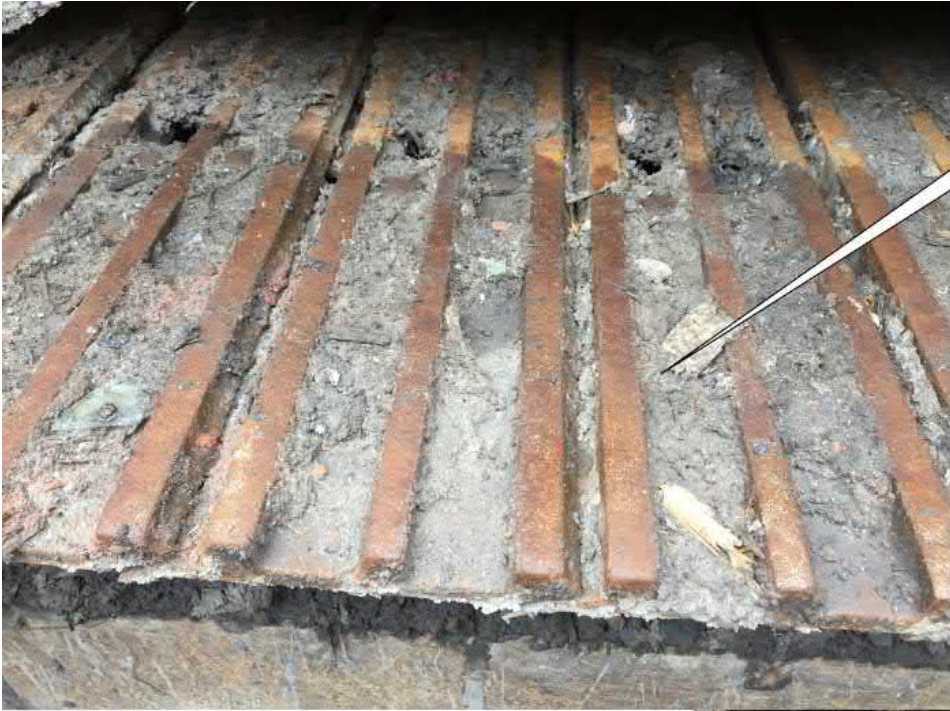
Debris in Tracks
